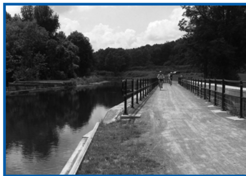
Results of the 2010 Canalway Trail Count estimated annual trail traffic of almost 249,000 persons at the Nine Mile Creek Aqueduct in Camillus.
